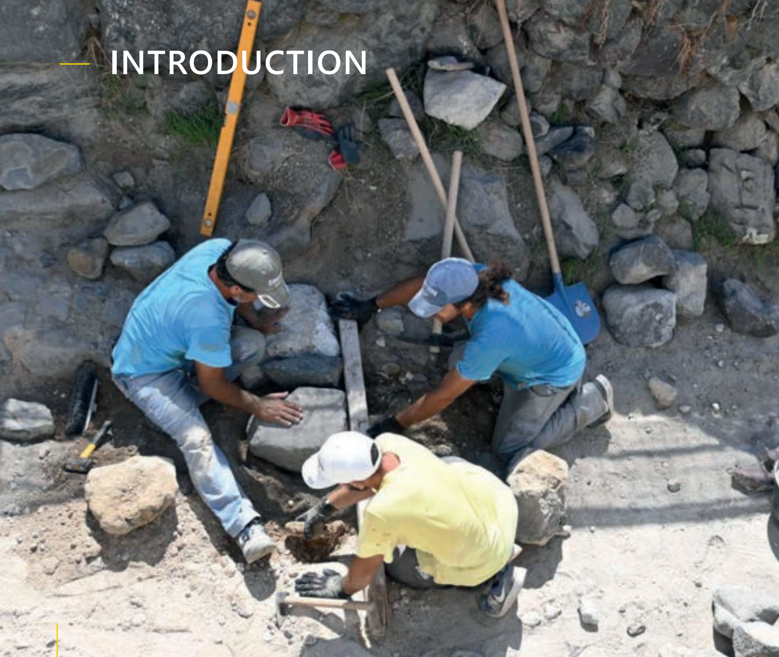
Trainer and apprentices while leveling the cobblestone during restoration works, Cyclades, Greece.
