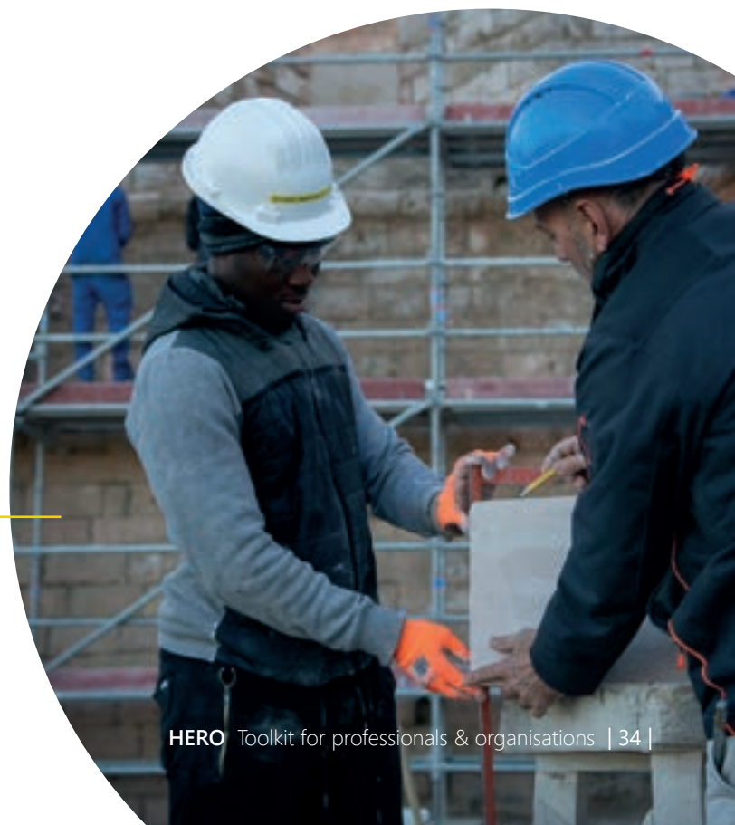
A trainer helping a trainee to mark stones for adjustments on the Fort St Nicolas worksite Marseille, France
