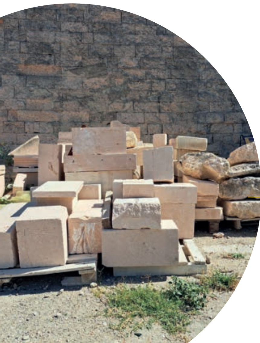
Stockpile of stones ready to be used on the Fort St Nicolas worksite Marseille, France
