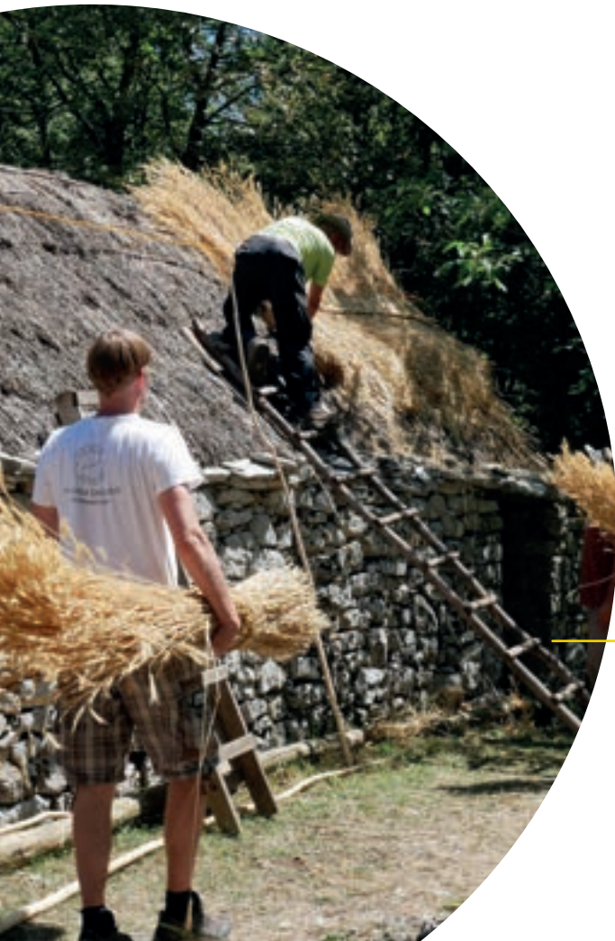
Restoring a thatched hay roof of a mountain shelter Petrebišća, Učka mountain, Croatia
