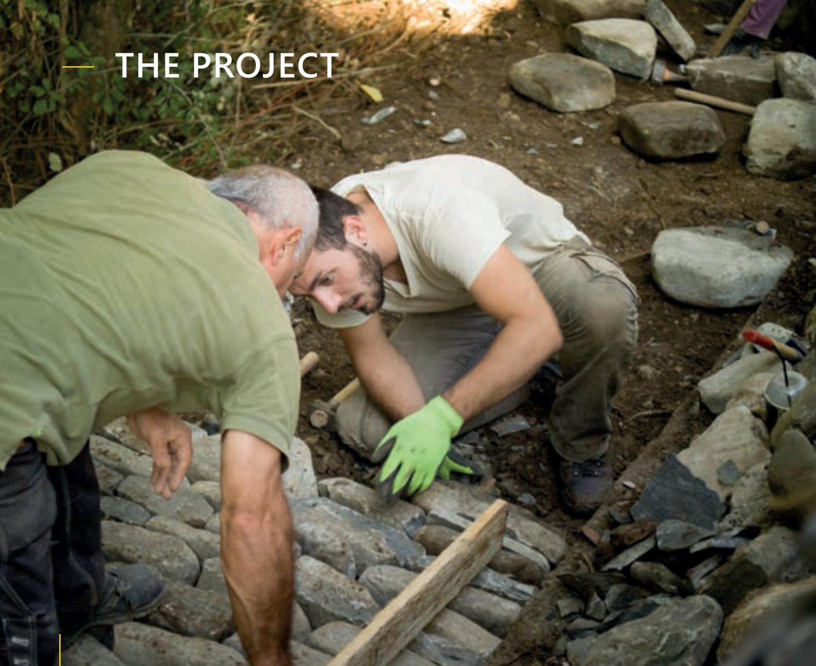
An apprentice guided by the craftsman on the construction of drystone pathway, Epirus, Greece.
