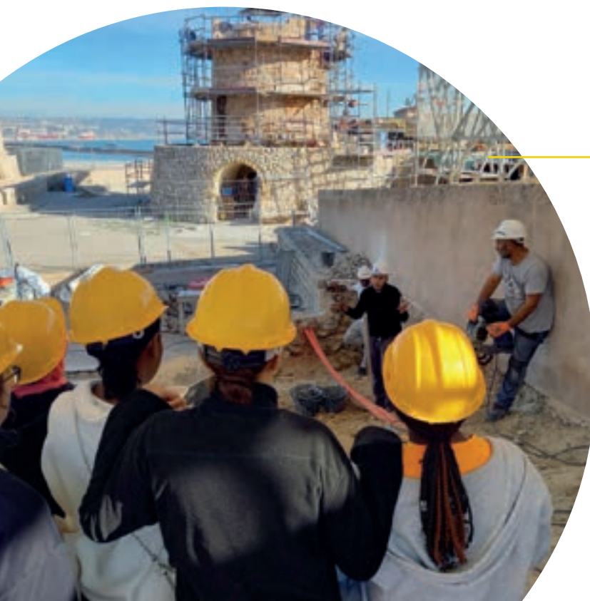
Trainees explaining their work to a group of kids visiting the Fort St Nicolas worksite Marseille, France
